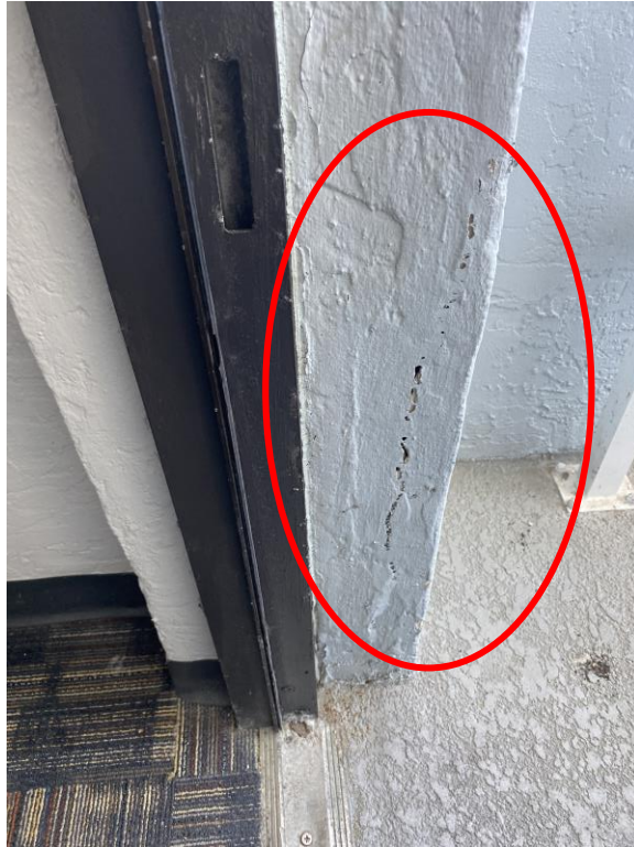
Photograph #11 – Typical walkway column spall at doorway
