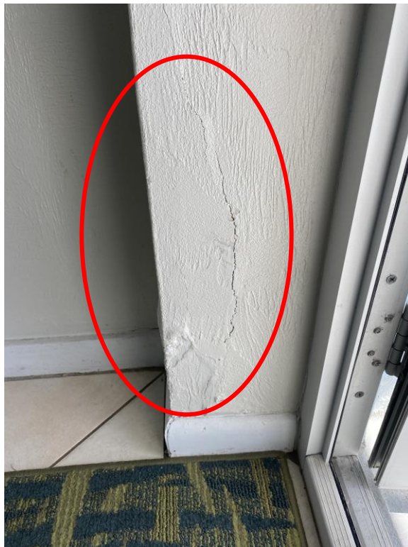
Photograph #12 – Typical column spall at unit interior
