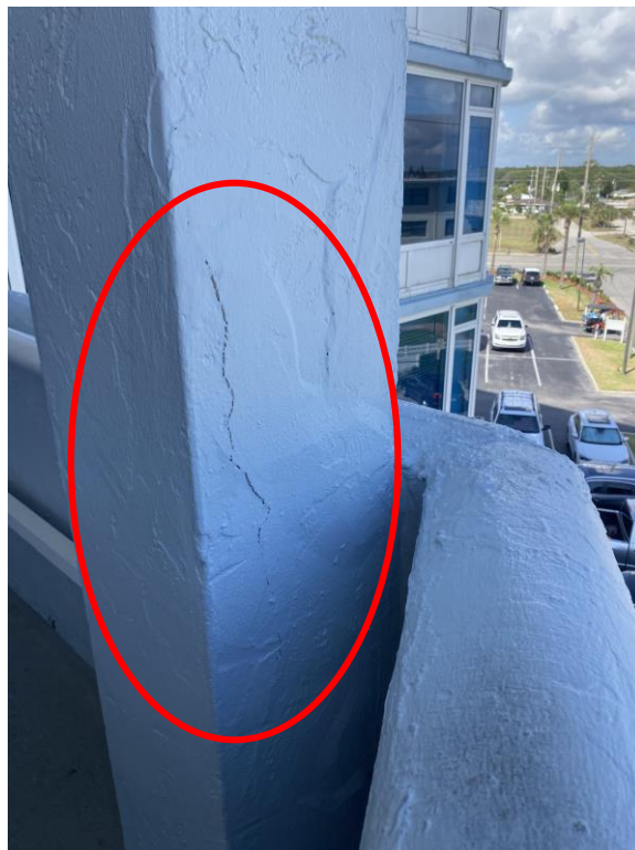
Photograph #10 – Column damage at North walkway recommended for immediate repair
