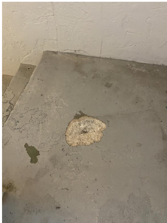
Photograph #8 – Typical top slab spalling damage
