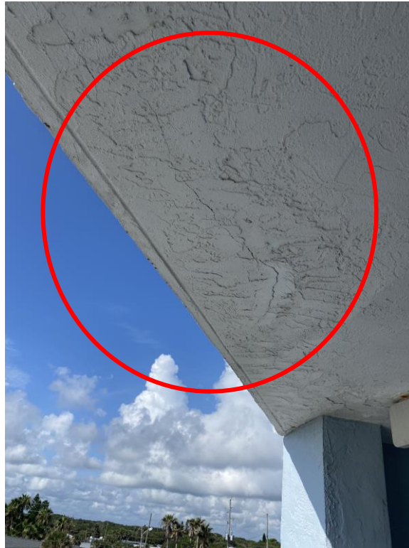
Photograph #7 – Typical slab edge crack at South walkways
