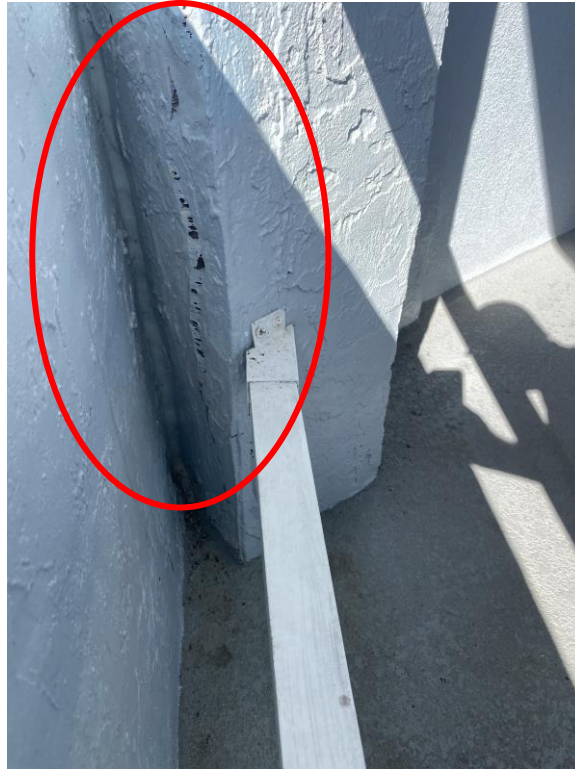
Photograph #9 – Severe column damage at South walkway recommended for immediate repair
