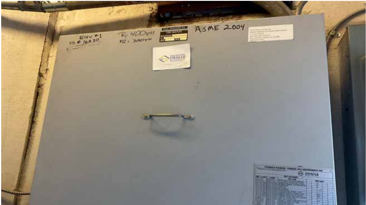
Elevator Equipment Rm North
