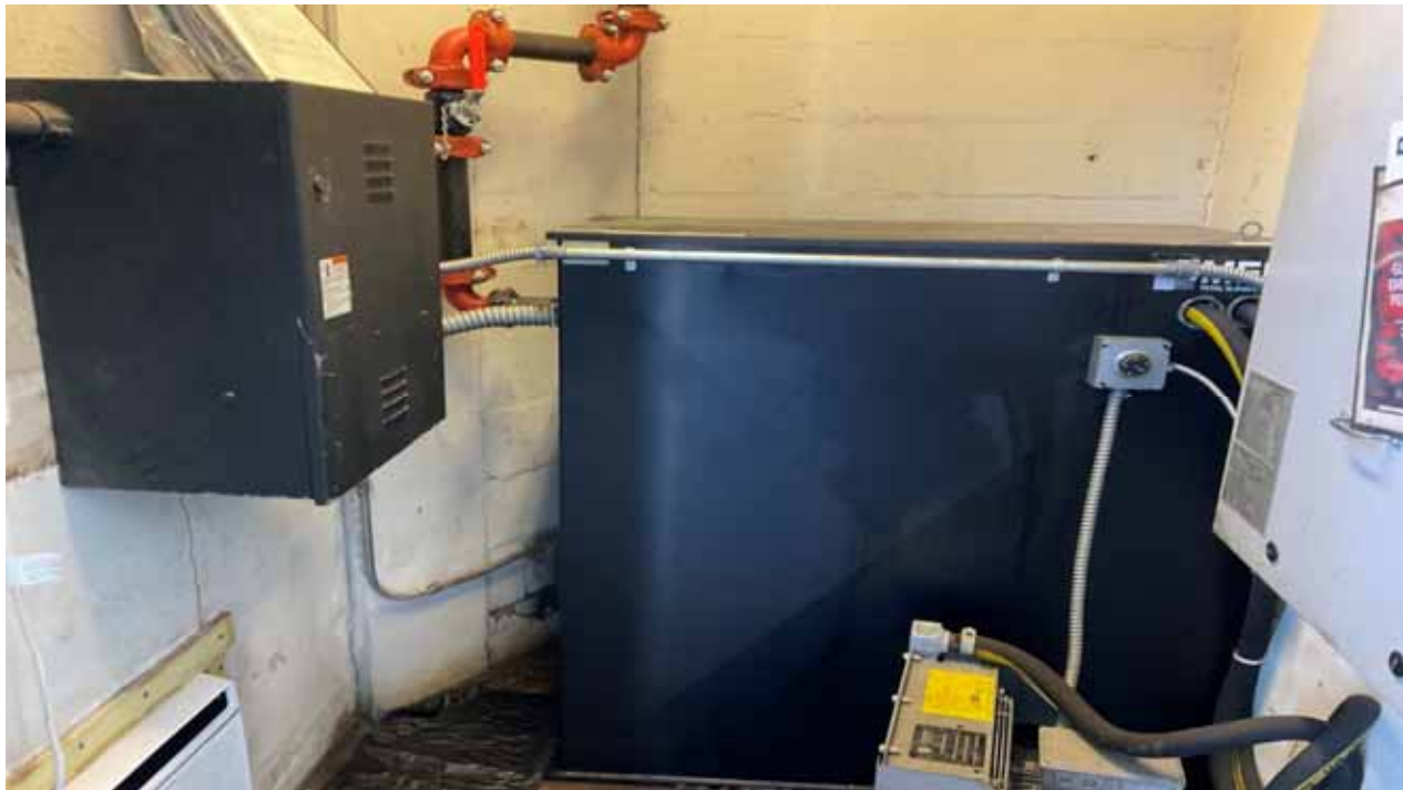
Elevator Equipment Rm South
