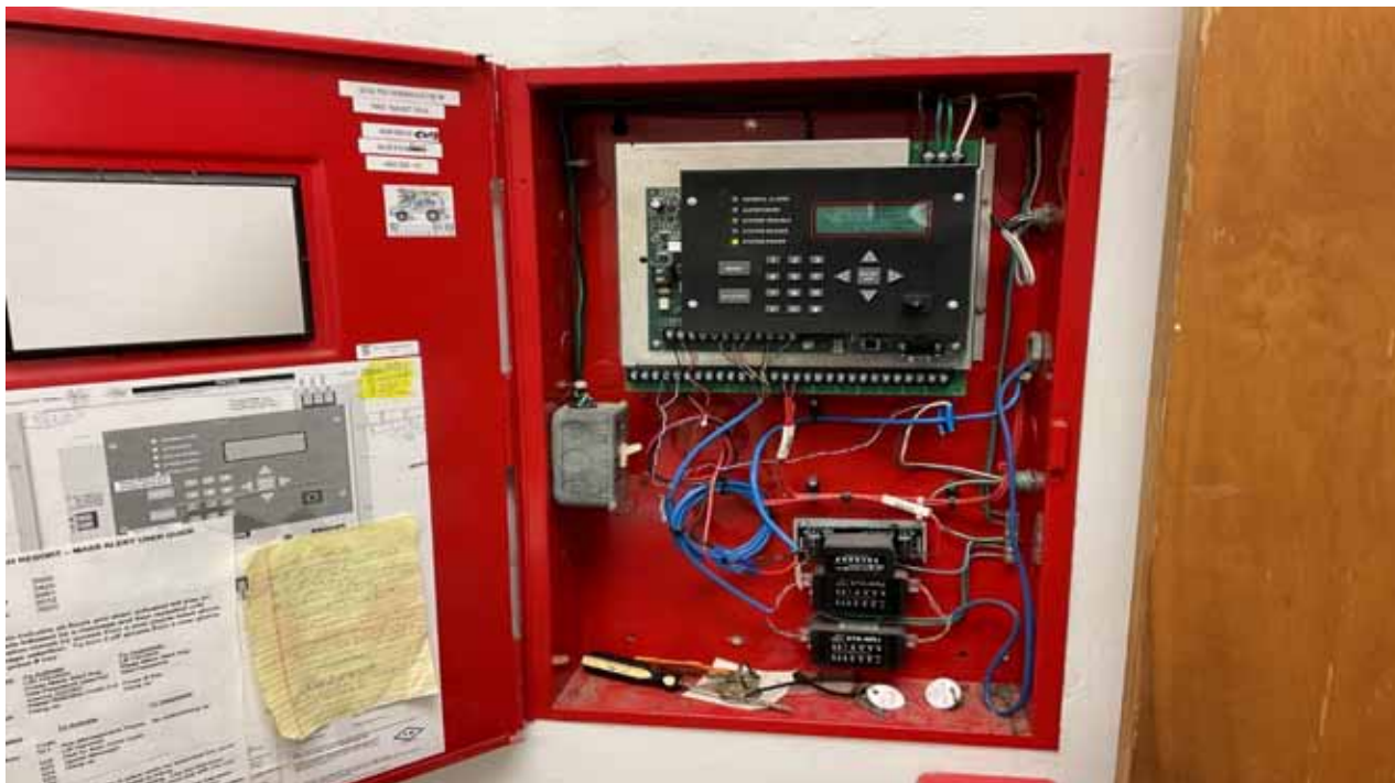
Fire Alarm Control Panel
