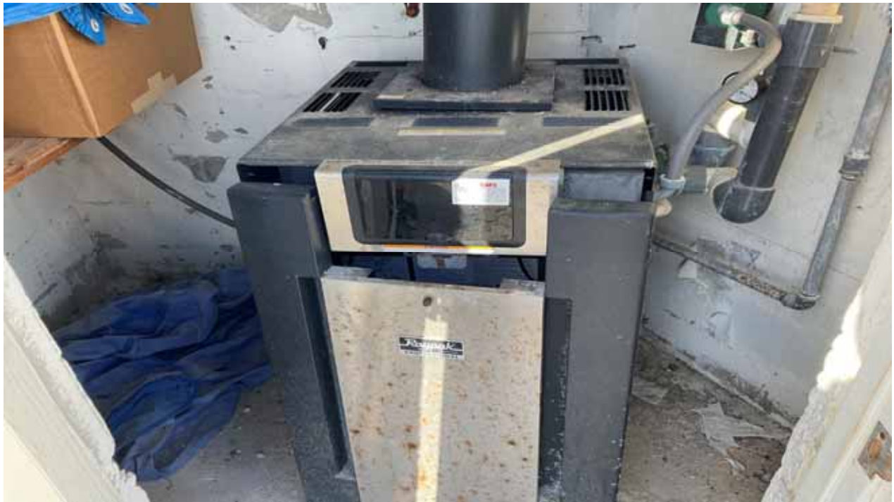
Spa Heater - North
