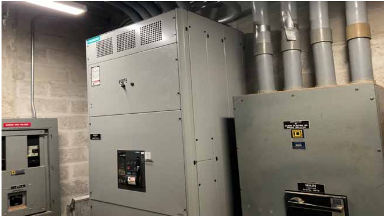
Main Electrical Room
