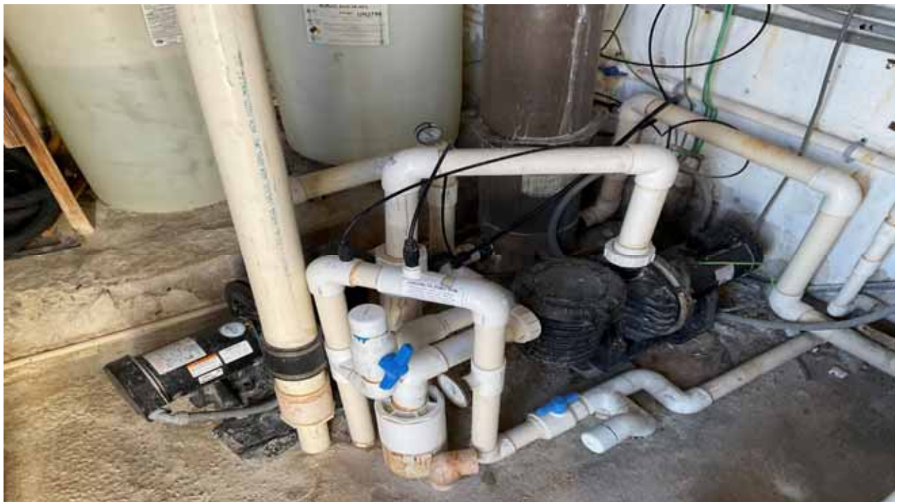
Spa Equipment - South
