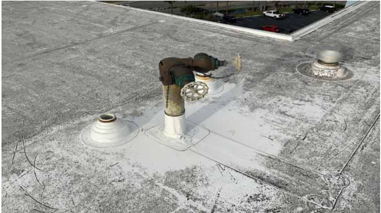
Roof - Sprinkler Riser
