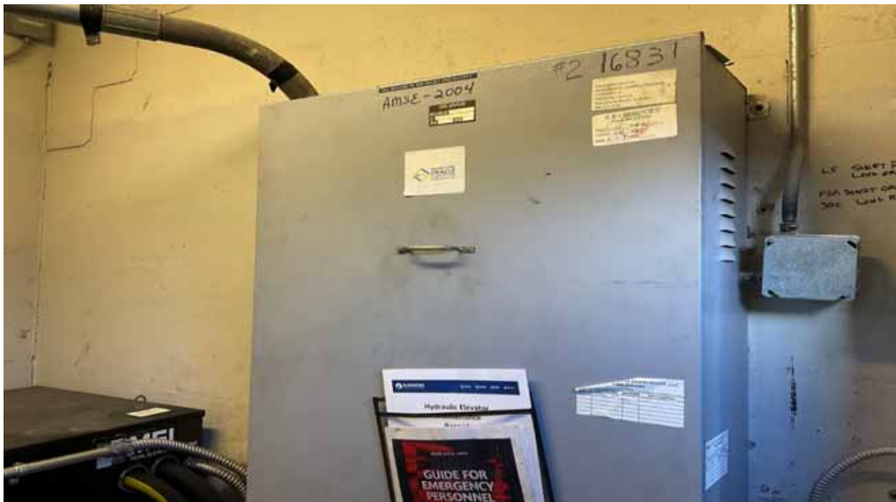
Elevator Equipment Rm South
