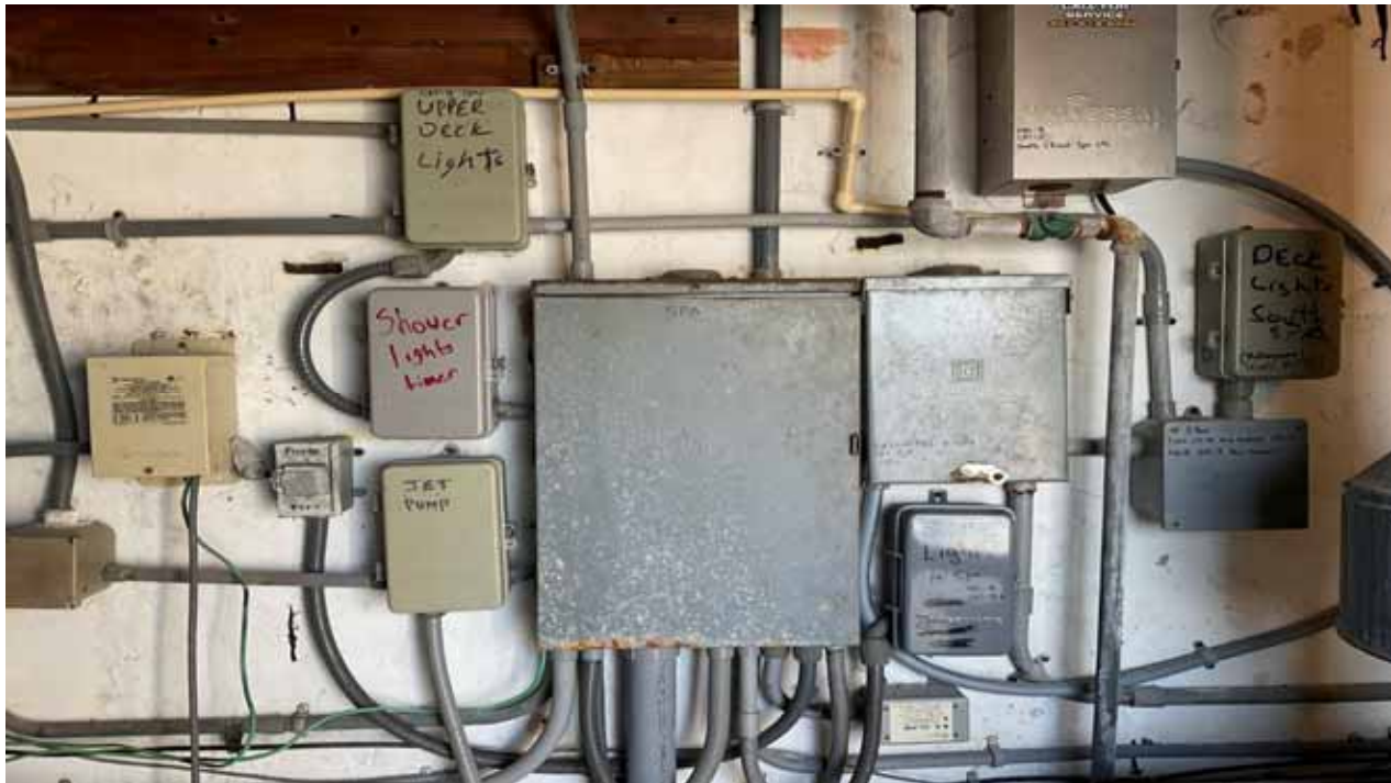
Spa Equipment - South
