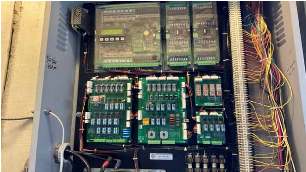
Elevator Equipment Rm North
