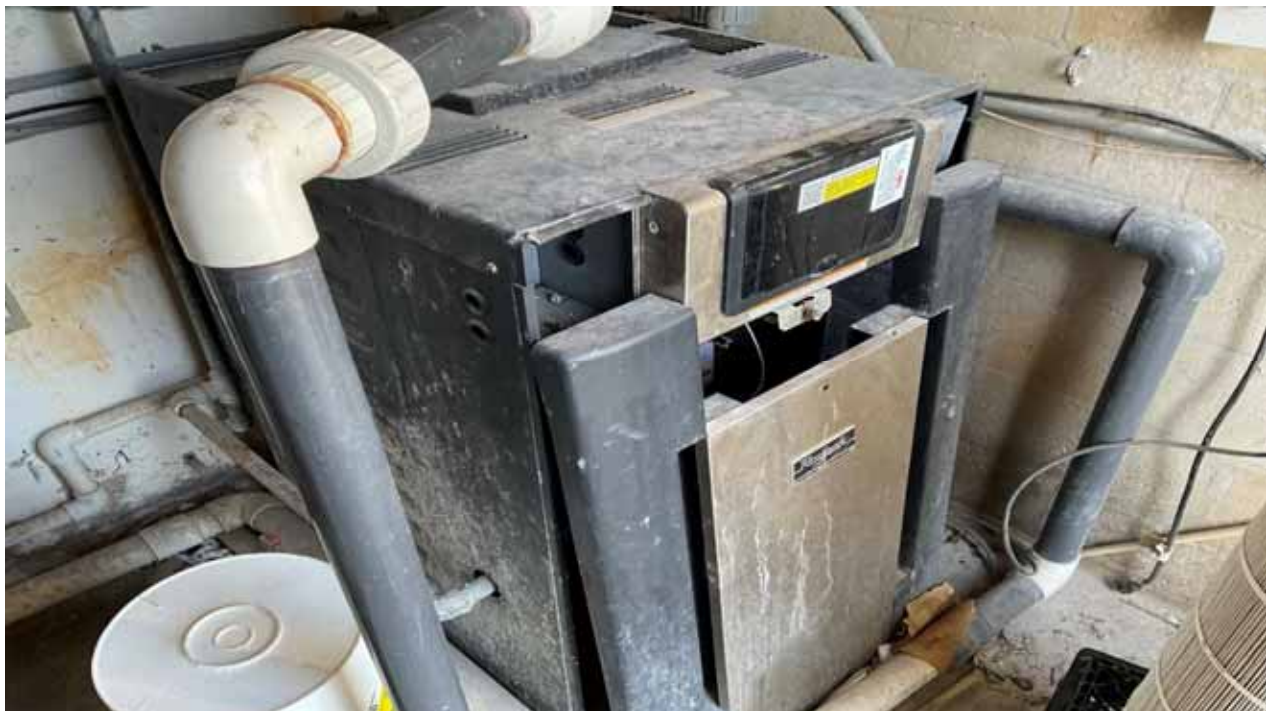
Spa Heater - South
