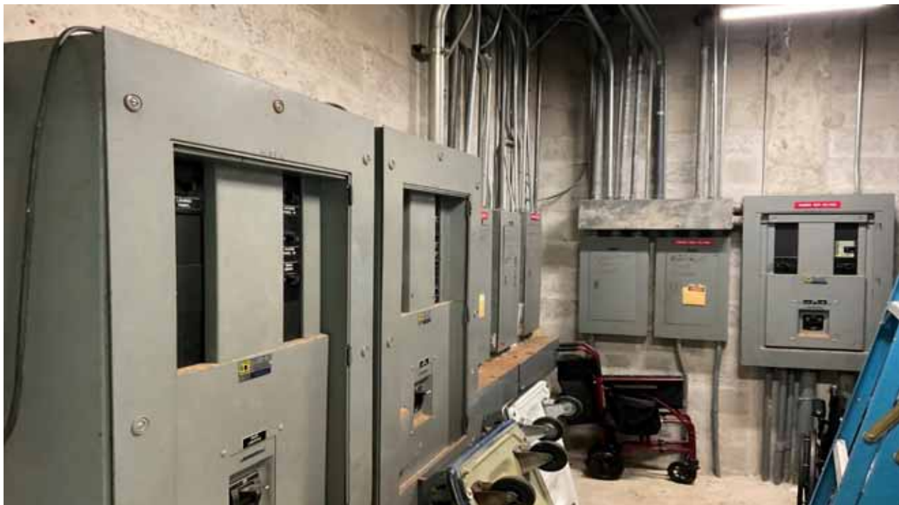
Main Electrical Room
