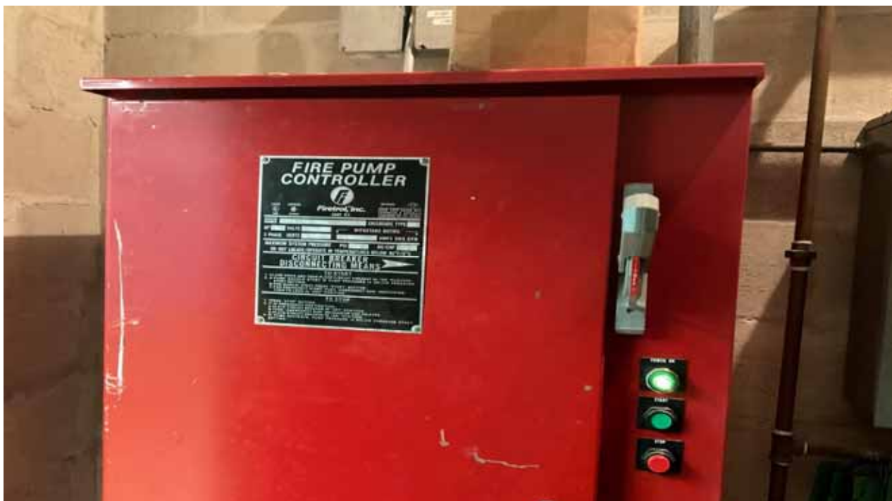
Fire Pump Controller
