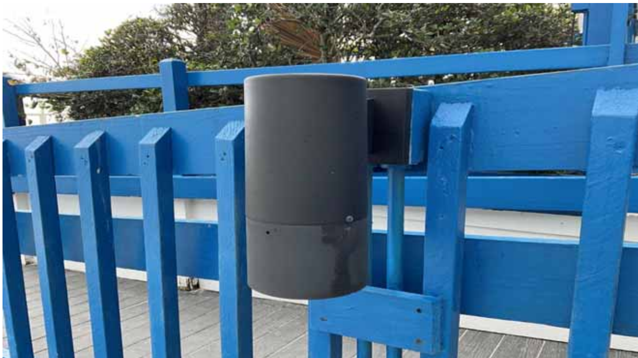
Lighting - Pool Deck
