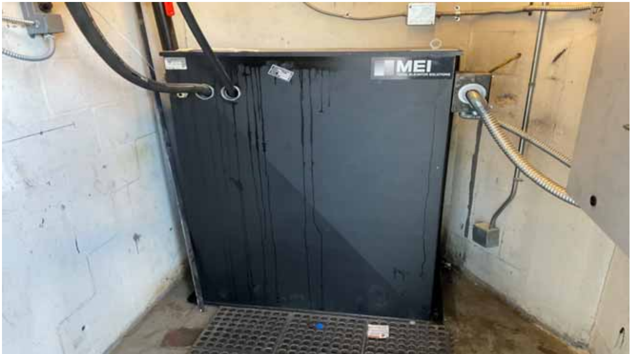
Elevator Equipment Rm North
